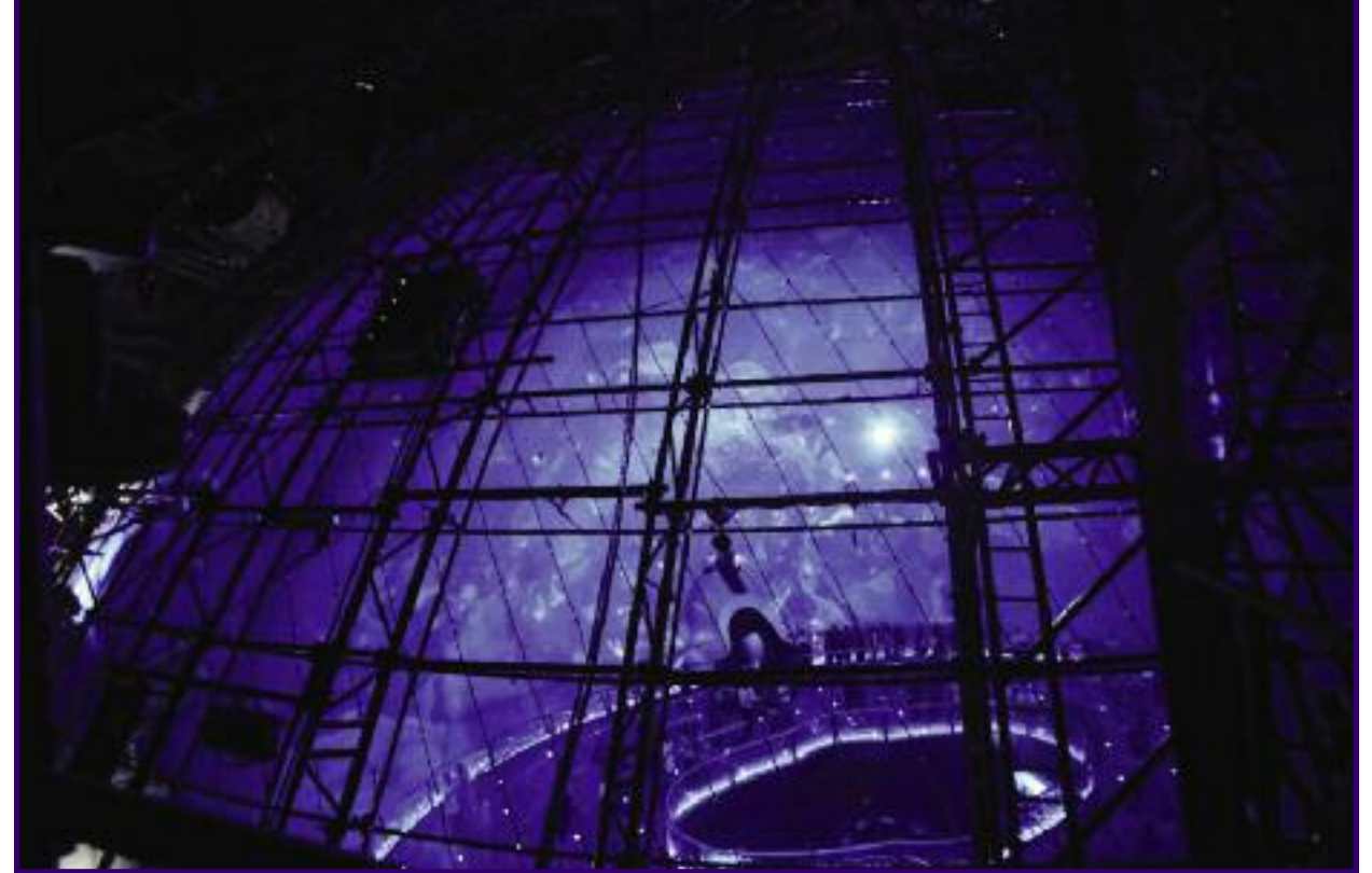
A view of the auditorium through the Bubble’s inner dome showing structural framework by Kraftwerk Living Technologies.
