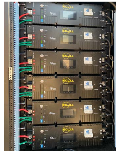
Battery technology has come a long way. Lithium iron phosphate (LFP) batteries have high energy density but are very stable and safe. They pose no hazard and have no cobalt.
