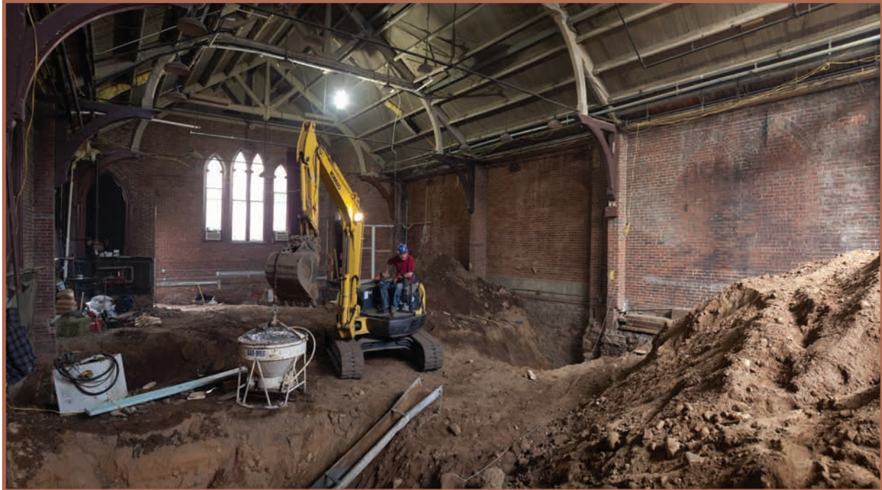
Because the building had no functional basement, the decision was taken to create one by gutting the interior, underpinning the building, and digging 14' into the ground.
