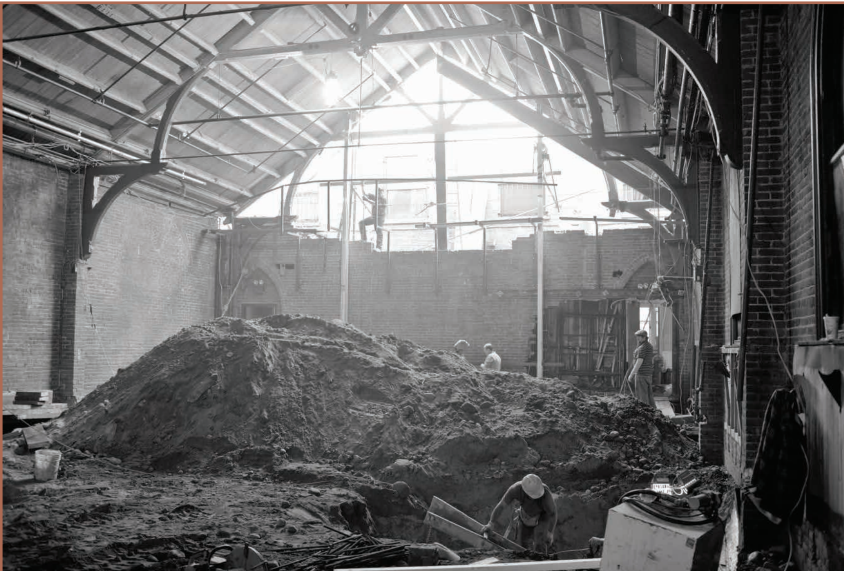
The effort of digging a basement for the theatre took seven months, but it resulted in 5,100 sq. ft. of basement space that now houses restrooms, a concession stand, a costume shop, a prop building shop, an IT room, and offices for technical staff.
