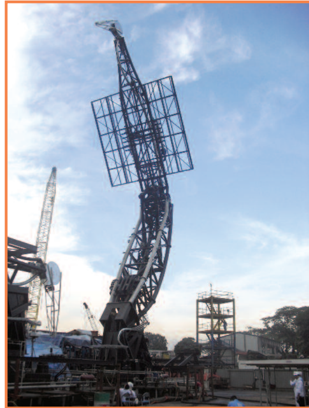
A crane under construction, with the frame for the video screen in place.
