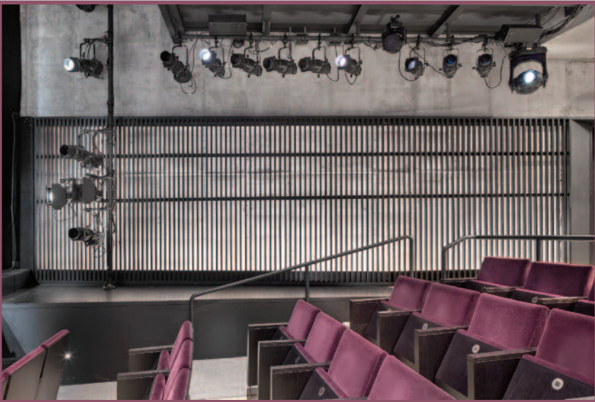
The Newman Mills has an exposed look, with plenty of hanging positions for gear. Gear for the audio-visual system was supplied by Masque Sound.
