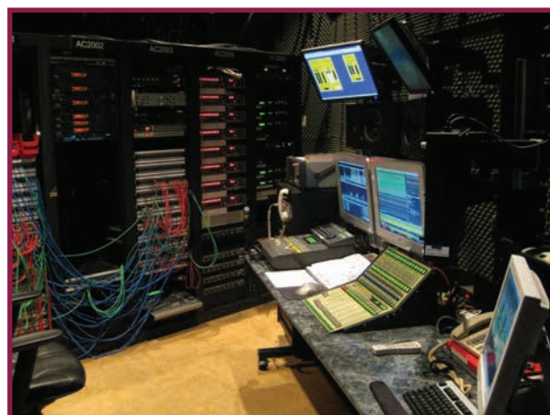
The backstage technical area housed a Meyer LCS CueConsole control surface and Matrix3 mixing system for monitoring.
