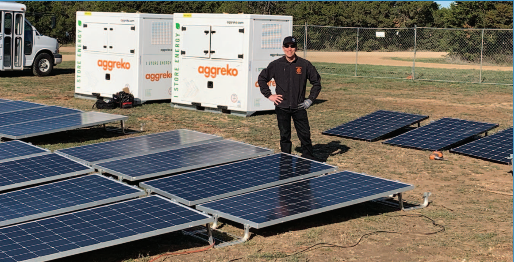
Posted online, this picture of solar panels and battery energy storage units elicited a range of responses from the live event community, mostly supportive, but some people were skeptical.
