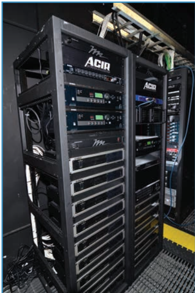
The theatre's AFC retrofit was completed with the assistance of ACIR Professional.
