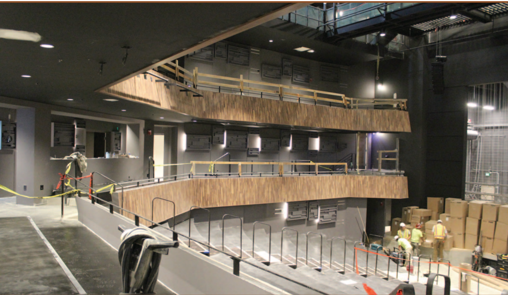
The theatre under construction. Much of the existing structure, including the administrative wing and lobby, was "reused and stitched back together quite successfully," Dachs says.
