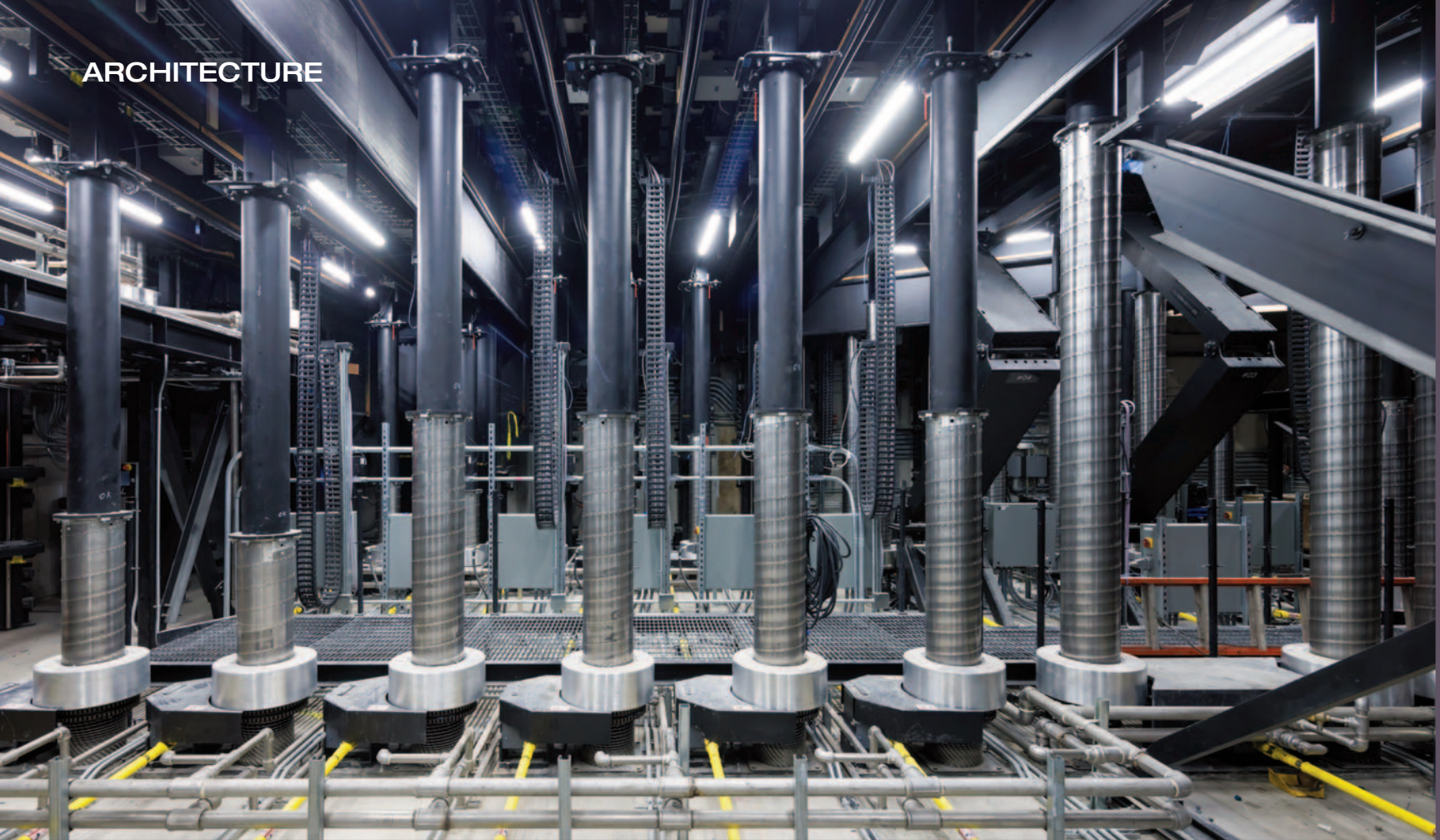
The mechanical room.
